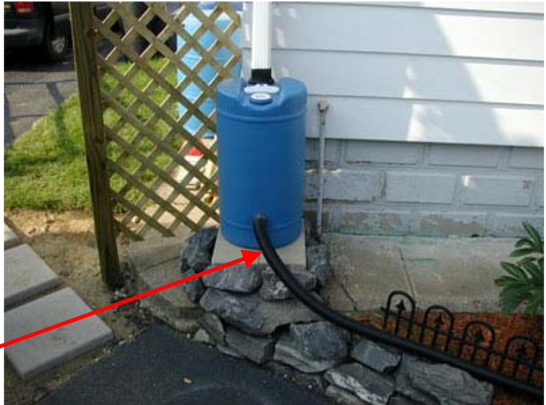
Sump Pump Hose
