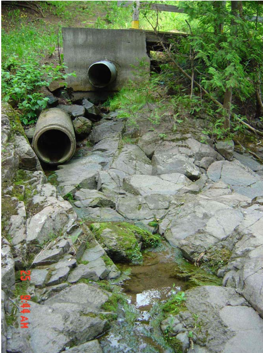
Fig. 4 Periphyton in stormwater inlet (Amity Cr.)
