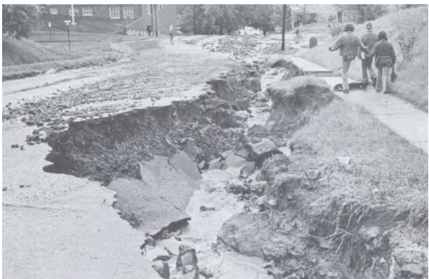
Washout of First Ave. East due to runoff
