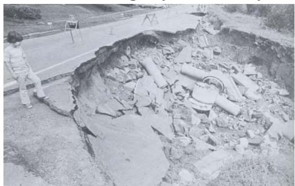
Stormwater inputs to Buckingham Creek along Skyline Parkway at 9 th Ave West
