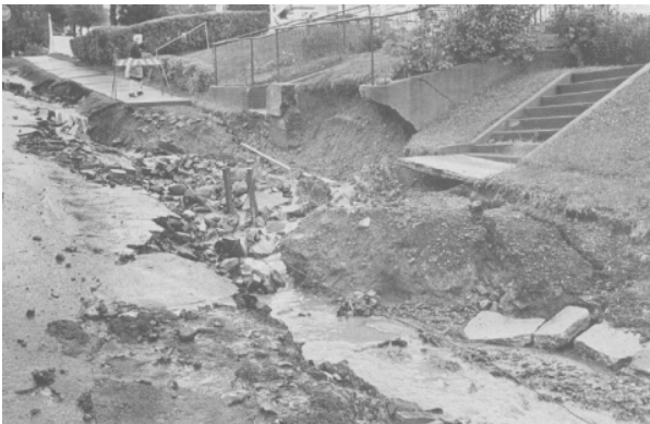
Washout due to runoff at First Ave. East
