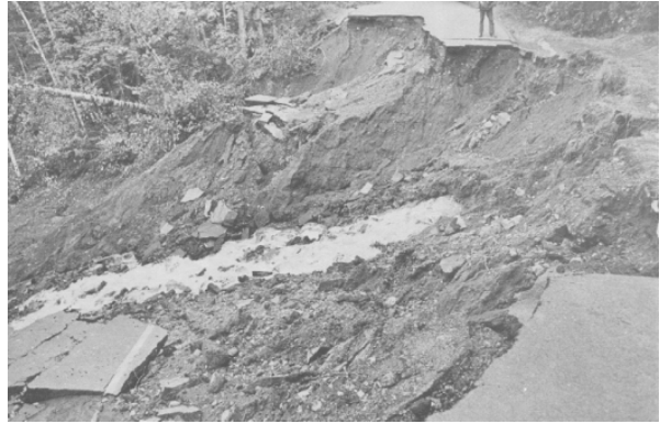
Washout along Skyline Parkway
