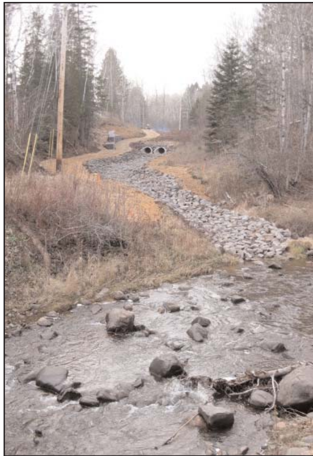
A rip rap rock channel now carries cleaner stormwater into Amity Creek and gateway to the Amity trails.
